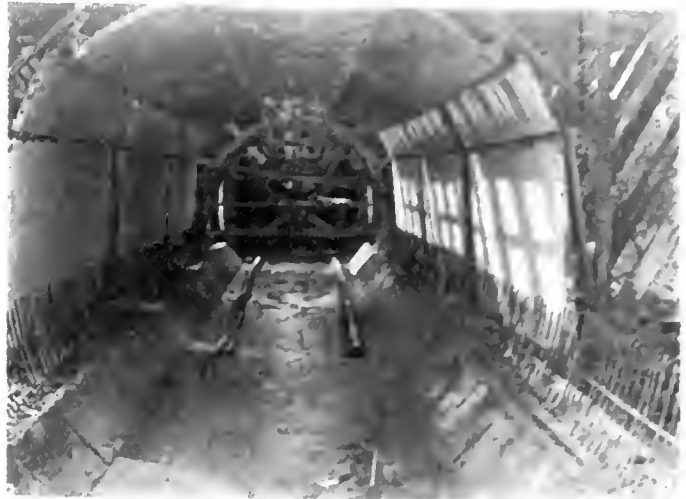
Invert completed and track laid for inner forms. Outer forms being placed. —Note reinforcing rods to join the invert to the superstructure.
